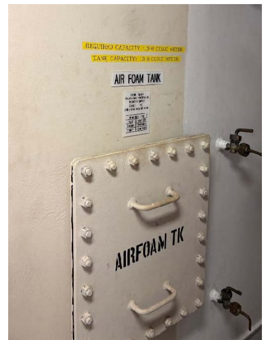
Foam storage tank – determines system endurance
