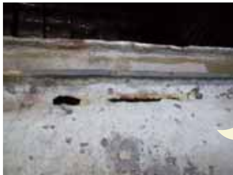
Photograph 12 Steel to steel achieved by contact between panel side plating and coaming table. Grooving and through corrosion in way of panel/coaming interface
