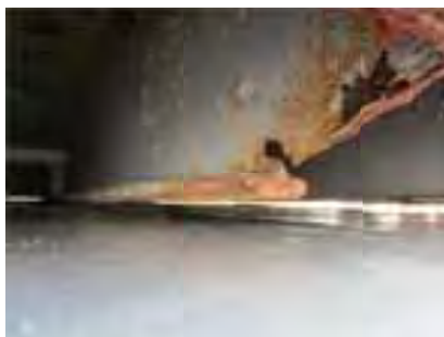
Photograph 4 Advanced corrosion to hatch panels
