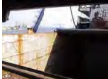
Photograph 7 Evidence of leakage traces on inner hatch coaming plating
