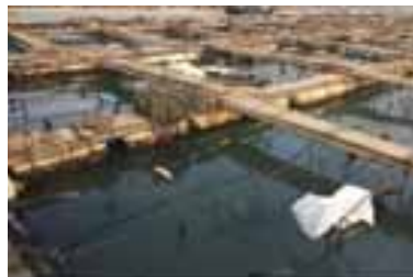
Photograph 37: Damage to Fishing Facilities
