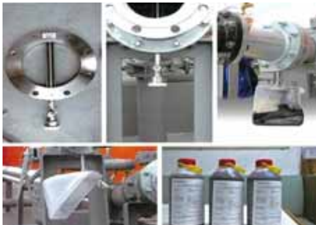
Photograph 5-33(b) Sampling of fuel oil
