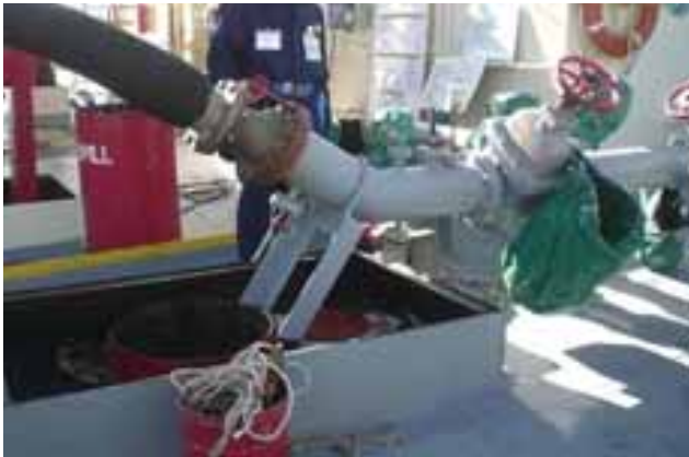
Photograph 5-33(a) Ship bunker manifold
