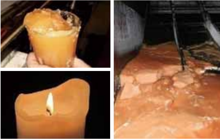
Photograph 5-22 Wax crystal formation in the fuel oil tank
