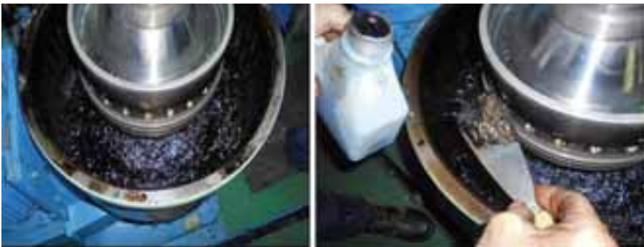
Photograph 5-9 Sludge deposition and precipitation within the rotating bowl of the oil purifier
