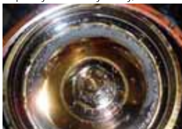
HFO separator : completely blocked by heavy, hard sludge
