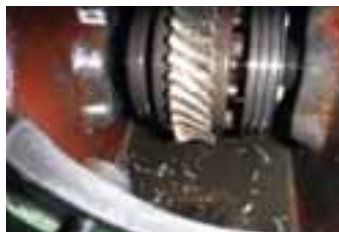
HFO separator damaged gear due to overload caused by heavy sludge
