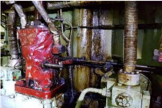
Serious fuel oil leakage from Main Engine
