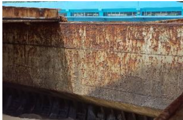
Cargo holds in extremely rusty condition
