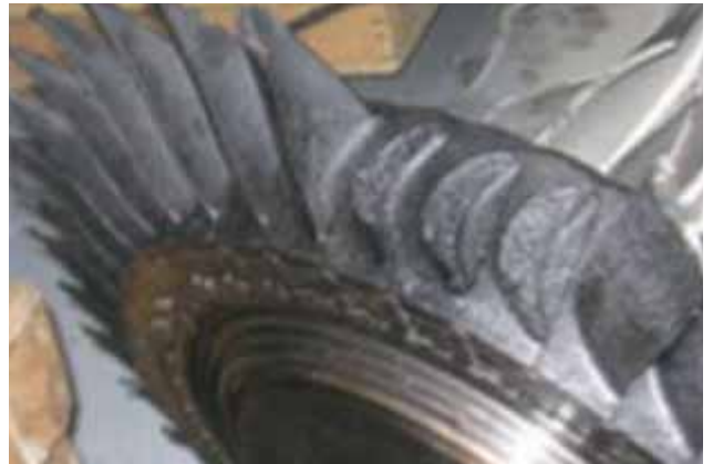
b) Broken turbine blade Damage leading to speed reduction in fiscal year 2014 / reference *4
