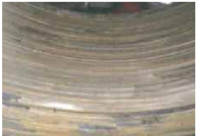
d) Burned-out intermediate shaft bearing metal (Over heated) Damage leading to speed reduction in fiscal year 2011 / reference*10
