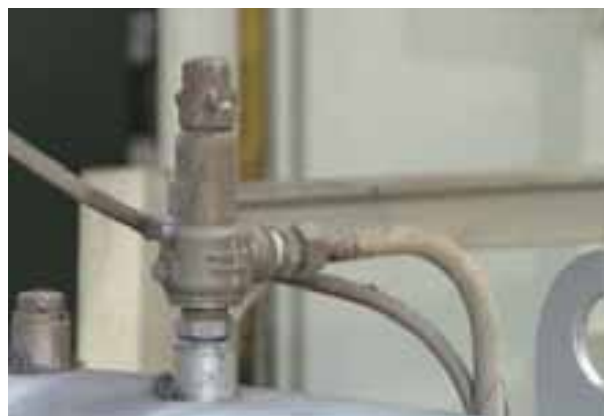
Figure 96 Leaking safety valve of fuel oil heater
