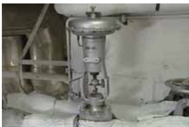
Figure 97 Damage of diaphragm on control valve
