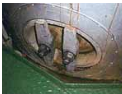
Figure35 Lower drum/manhole (Water leakage trace from upper part)
