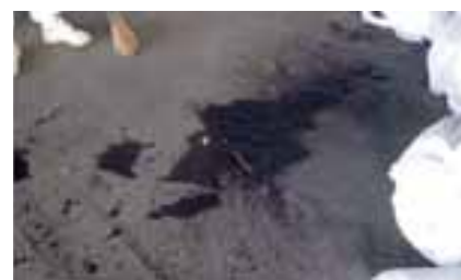
Figure 63 Soot on working passage inside factory
