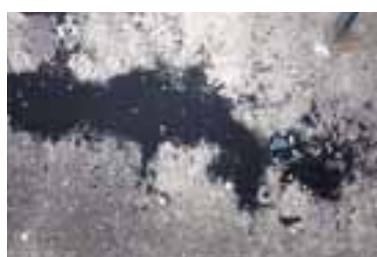
Figure 62 Soot on working passage of factory
