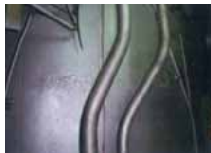
Figure36 Upper boiler casing (Paint swelling)
