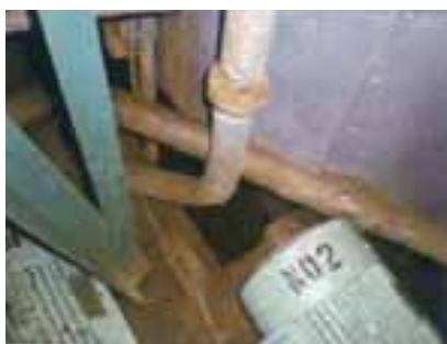
Figure34 Lower boiler casing (Water leakage trace from upper part)
