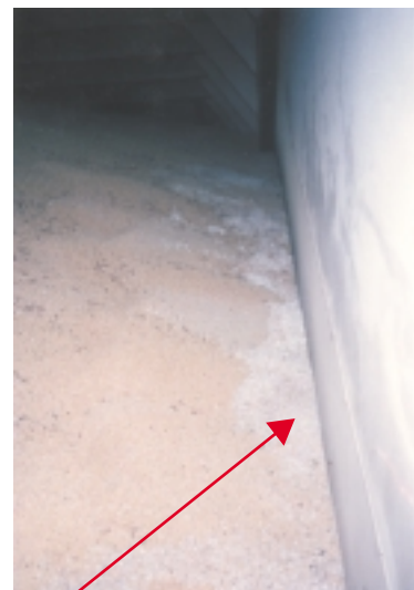
Mouldy cargo in the top surface along the aft bulkhead of the aftermost hold
