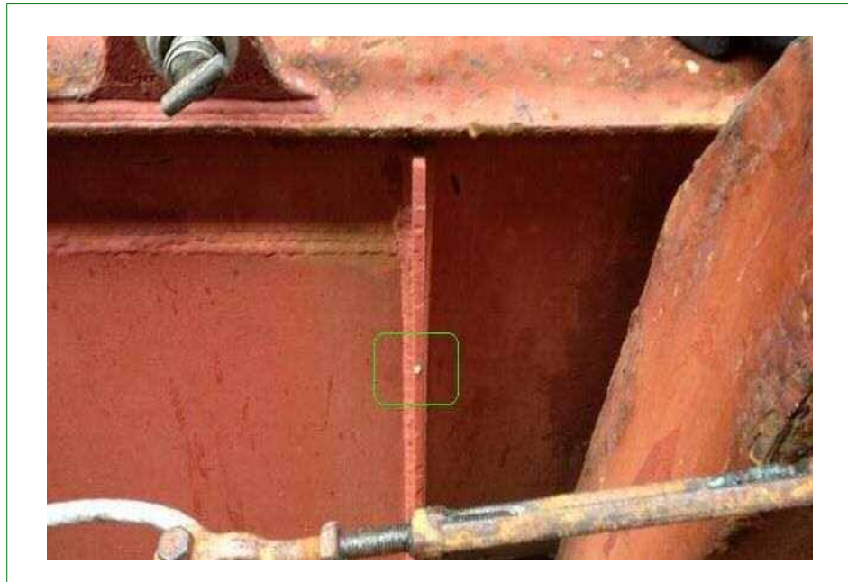
Figure 2 AGM Eggs Found Between Two Bays on a Support Beam Near a Cargo Hold Opening
