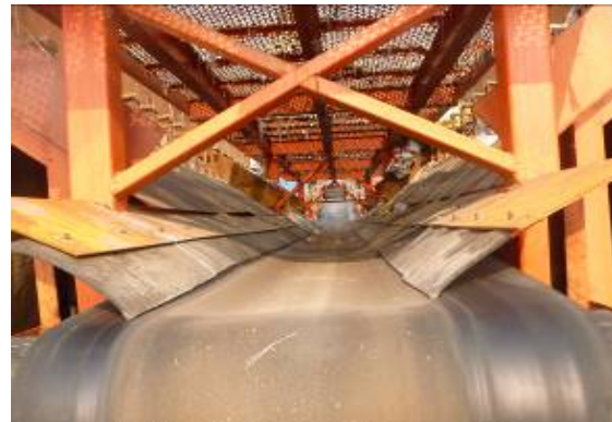
The fertilizer will drop on the conveyor belt over the iron griddle via the iron griddle
