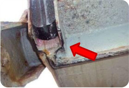
Example of recommendation: Rubber gasket partly missing
